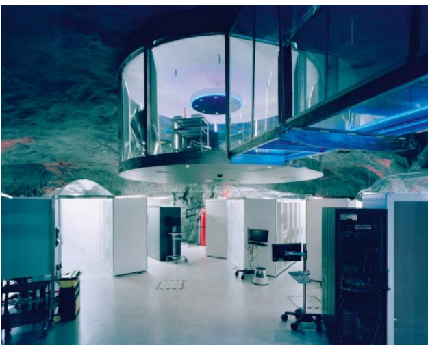
o5_High-security data center, Stockholm, Sweden, 2023 © Gregor Sailer
